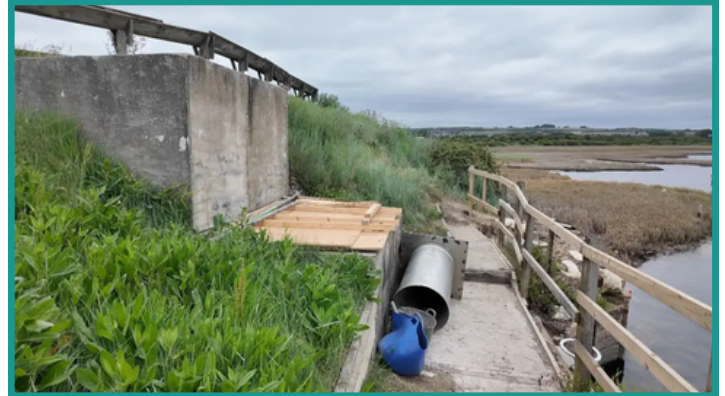
Sluice Gate, Farlington Marshes. © Environment Agency
